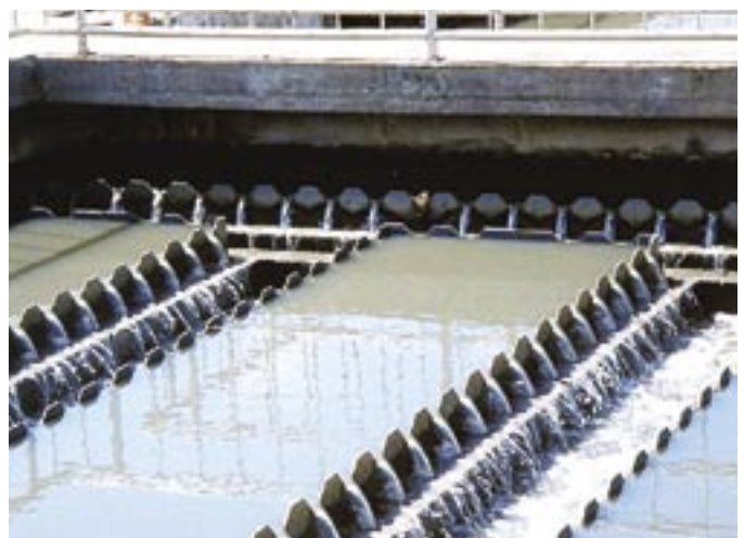
Notched Weir Plates
