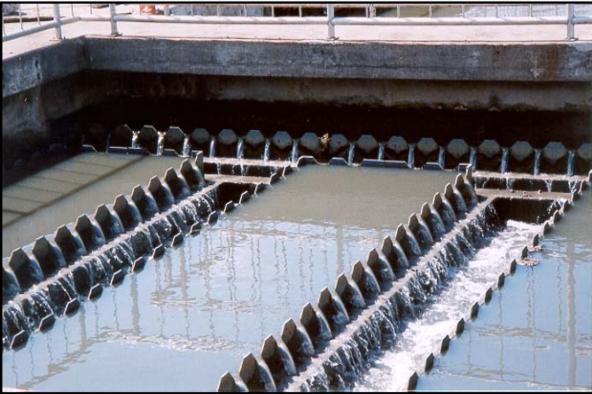
Factory built corners helped reduce leakage and improve efficiency after refurbishing weir plates at a sewage treatment plant in Hamilton, Ontario.
