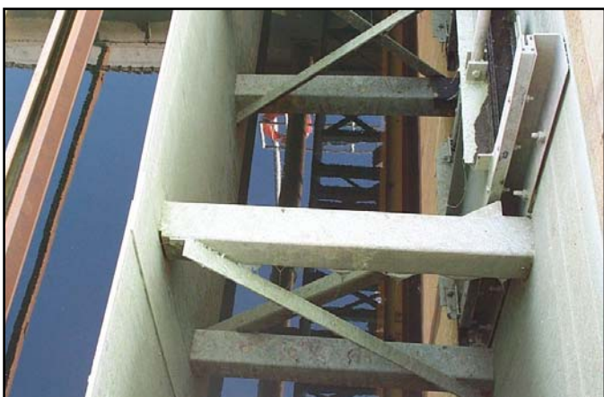
Inflow gate baffles used during tank fill operations provide excellent corrosion resistance and long service life.
