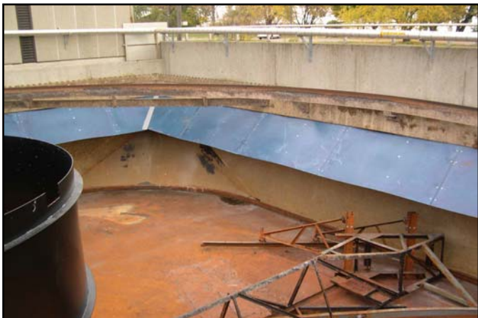
Current flow baffles installed in clarifiers at Burlington, Ontario have the added benefit of long lasting PCL mounting brackets to complement the FRP baffle plates.
